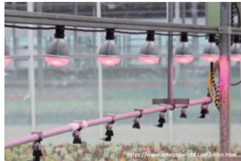
Lights on moving irrigation boom
